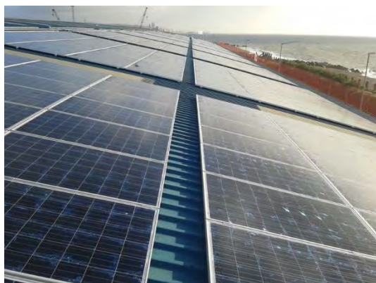
Solar panels on warehouse roofs
