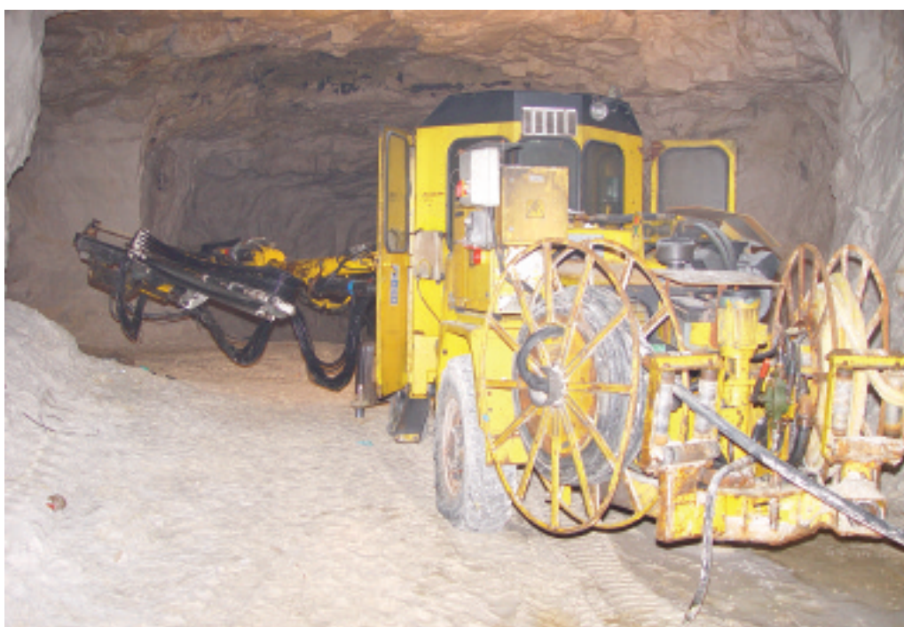
Blasthole drilling is carried out by an Atlas Copco H282 Boomer rig
